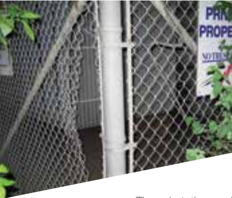
The substation yard where the thief broke in, attempting to steal copper. (Source: EPCOR Utilities Inc.)
