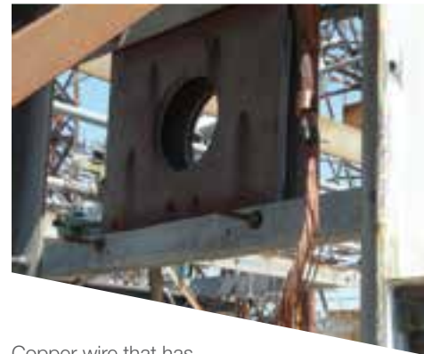
Copper wire that has been tampered with at an electrical substation in Ontario.
